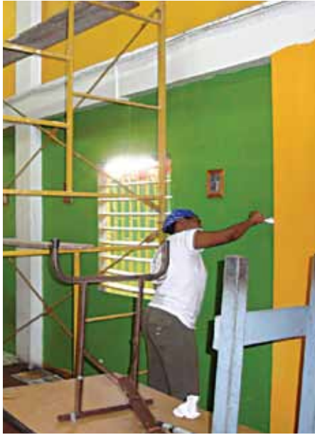
Volunteers of Atlantic LNG painting the interior walls of the Duncan Street Caring Facility.
